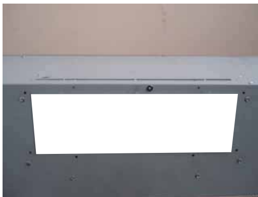
Horizontal Ducting (3-1/4"x10" Rectangular)
